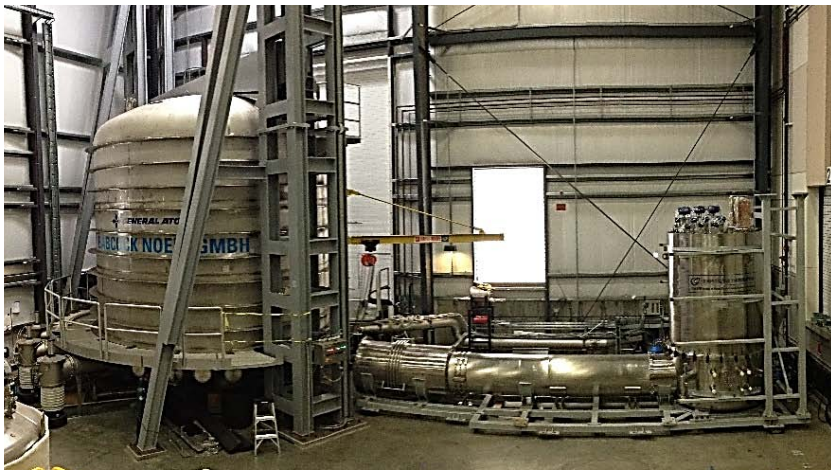
Test chamber and feeder installed at GA
