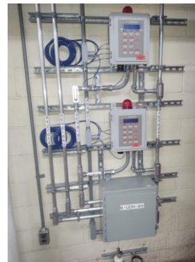
Redundant Alarming ODH Monitors
