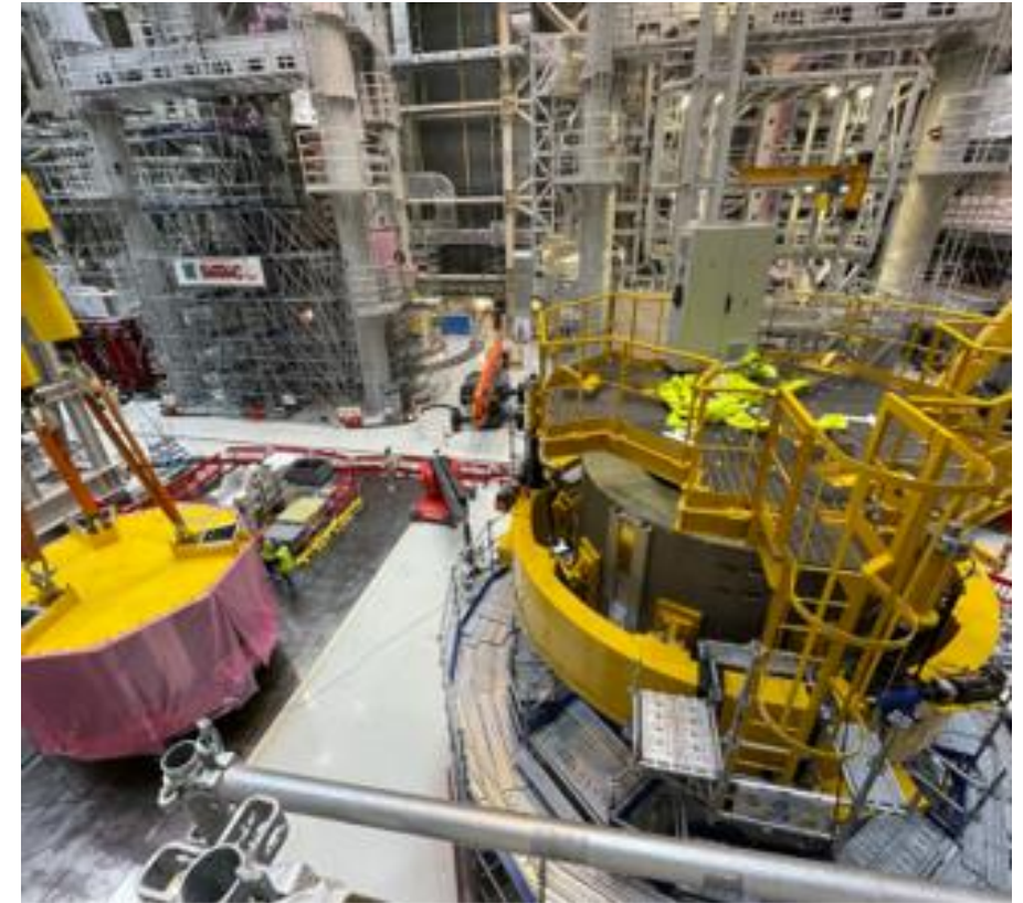
Overhead view of module #1 on the base and module #2 (wrapped in pink plastic)
