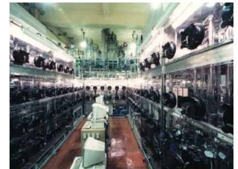
Tritium Plant system
