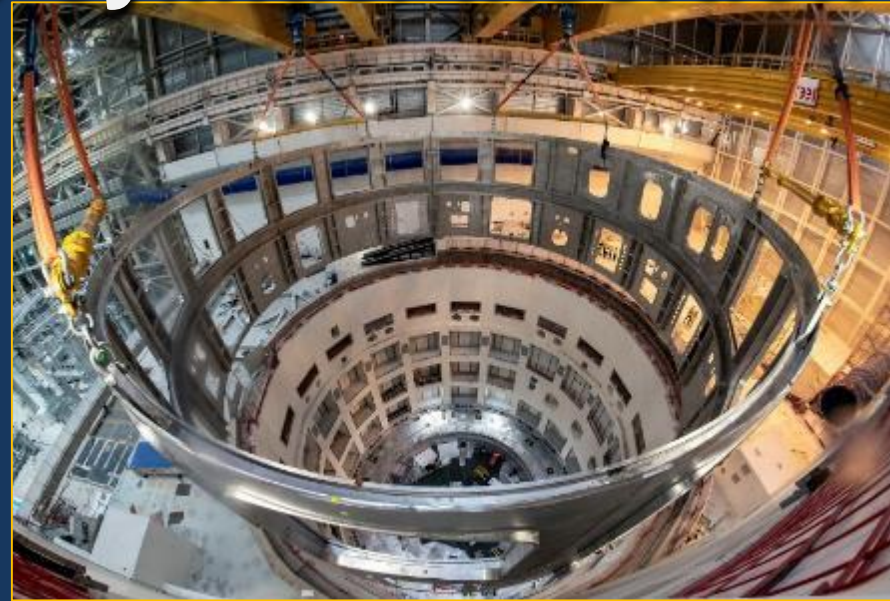
Inserting the Cryostat Lower Cylinder into the Tokamak Pit. Perfect fit with the Base 31 August 2020
